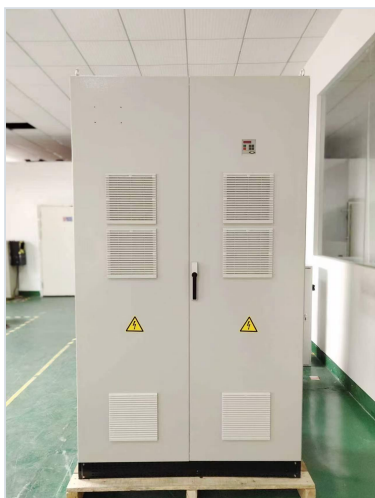
Front View — Installed Unit
