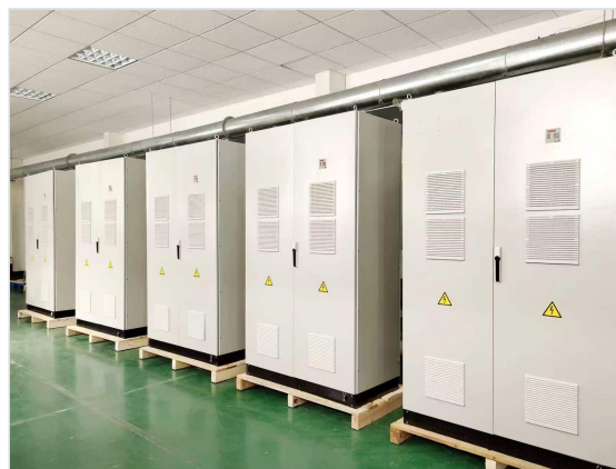
Cabinets Ready for Shipment
